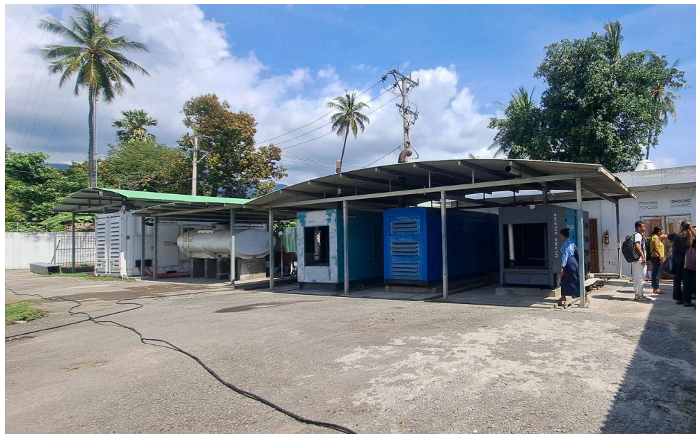
Figure 13. Backup generators in HNGV
