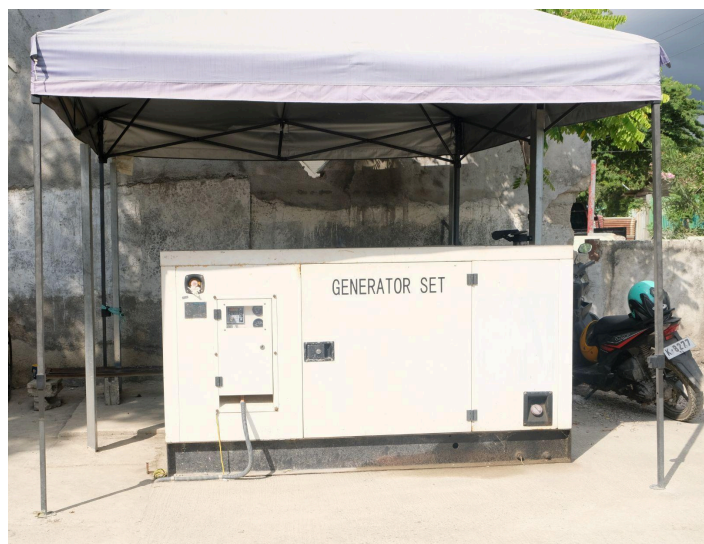
Figure 18. Backup generator set in CHC Comoro
