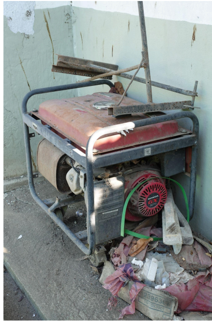
Figure 21. An unused generator at the Covalima Community Health Center
