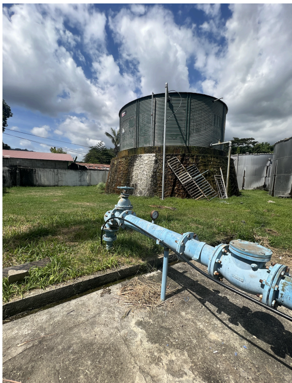
Figure 11. Water supply system in HNGV
