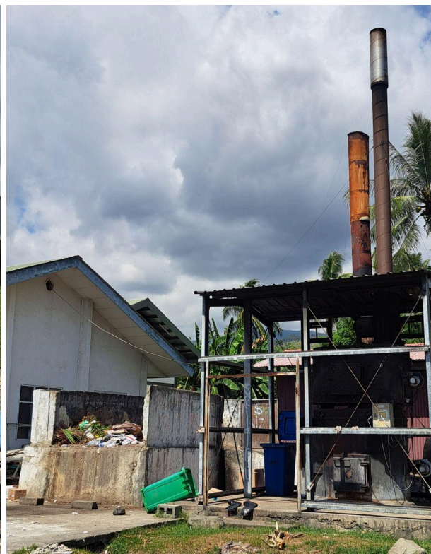
Figure 12. Medical Incinerator in HNGV
